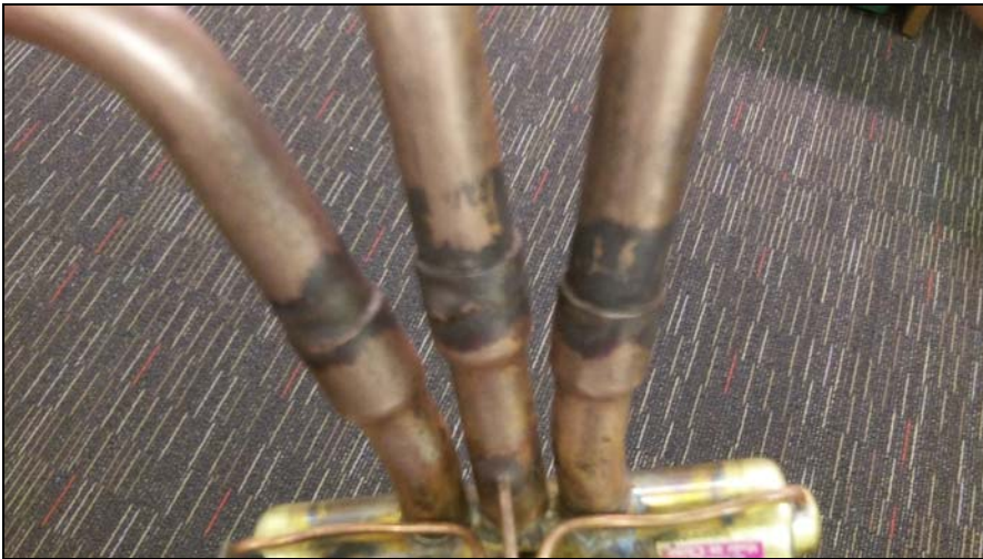
The three copper tubes and the braze joints
